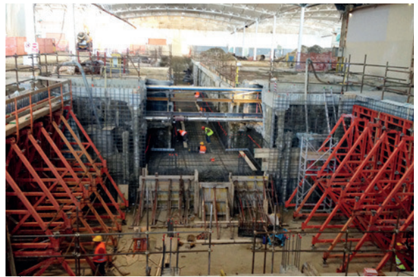
Tunnel TRUCK stabilimento PIRELLI, Settimo Torinese (TO) TRUCK tunnel, PIRELLI plant, Settimo Torinese (near Turin)
